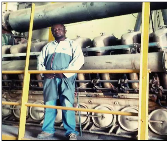
Fig 1: 3MVA Cockerill Generator Prime Mover
