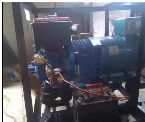
Fig 2: 5kVA Diesel Generator Assembled
